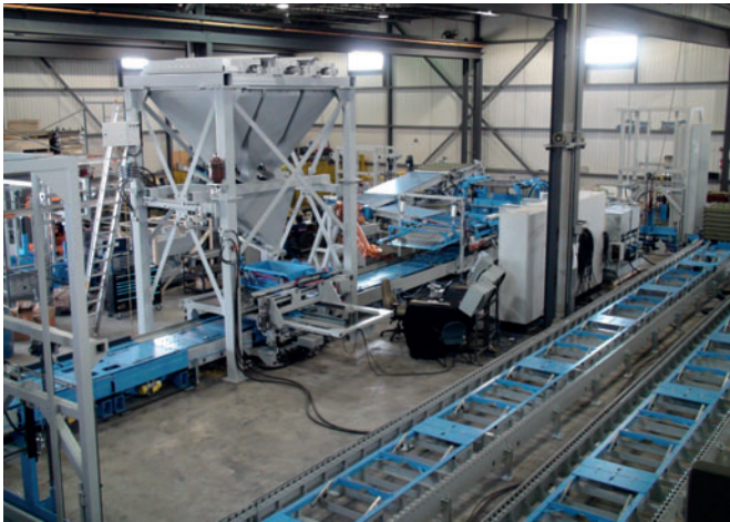
Fig. 3: An entire wet cast automated production plant for alternative masonry can be seen in this photo, including conveyor lines, automated filling stations, stacking and destacking, and other production equipment.
